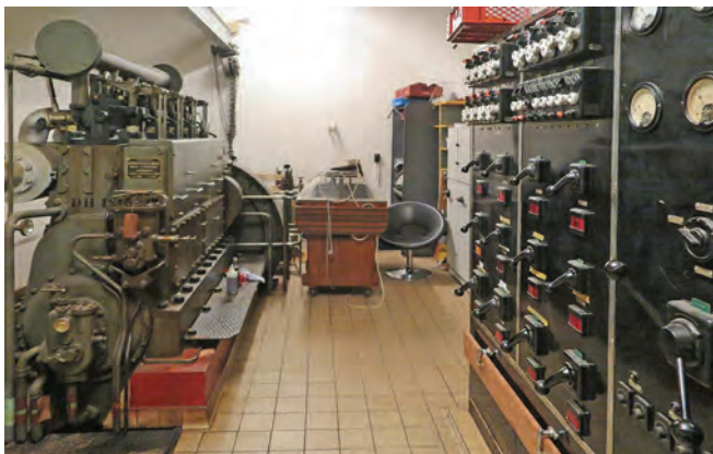
Generator and switchgear within Dragør Fort
